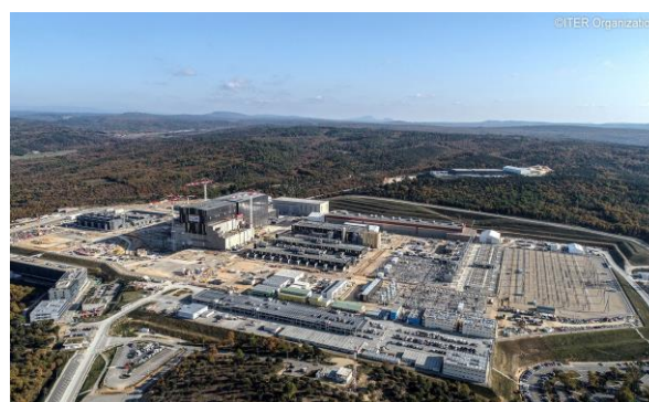
Construction of ITER (International Thermonuclear Experimental Reactor) in November 2020 (Cadarache in Saint-Paul-Lès-Durance, France) Source: ITER Organization
