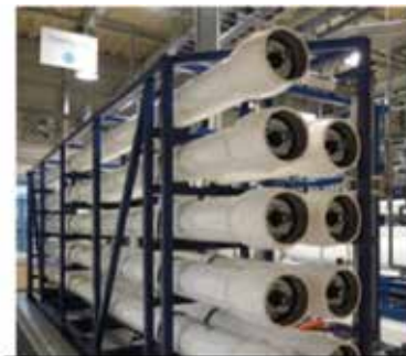
RO membrane system used in the “RemixWater” system
