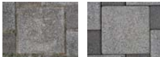
Before decontamination After decontamination *Decontamination was implemented with ultrahigh pressure water technology on a road surface which had revealed no decontamination effects when measured by the conventional method. Radioactive substances in gaps between blocks were removed. Courtesy of JAEA
