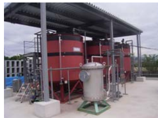
Ex. 5. HTCF-regeneration plant and phosphorus-recovery plant
